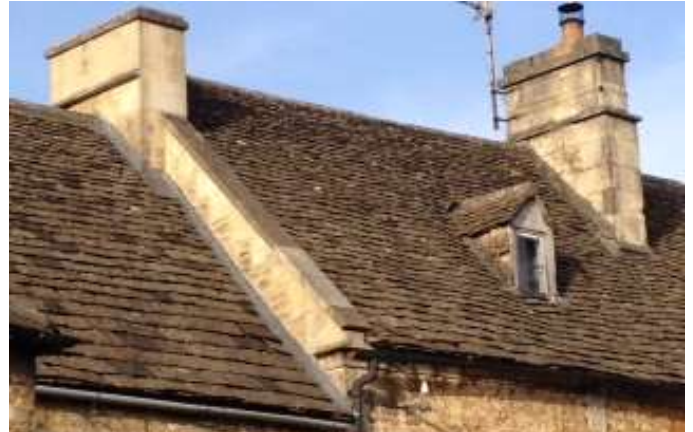
Rebuilt chimney stump (at left) but no shaft
