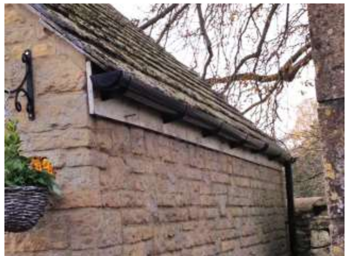
'fascia boards should not be used for fixing gutters'
