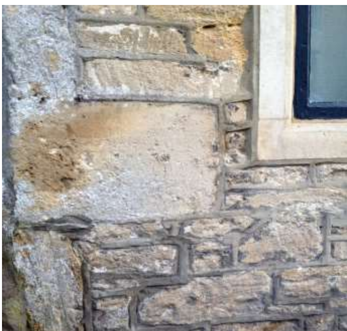
Cement rich ribbon pointing in Pickwick Street
